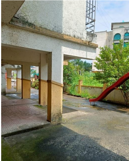
PICTURE 1: FUNGUS ALL OVER THE GROUND FLOOR, NO PROPER CLEANING MEASURES.
